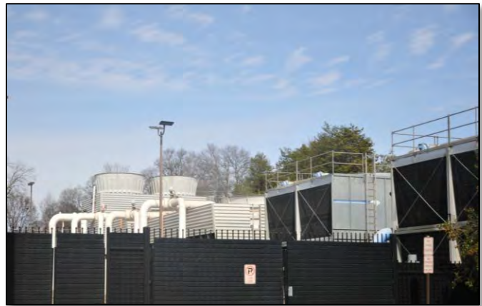
Figure 11: 10th Street Chiller Plant
